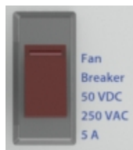
Figure 13. Fan Power Breaker
