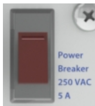
Figure 31. Power In Breaker
