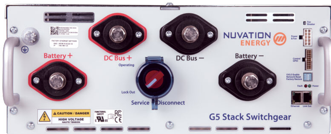
Figure 26. G5 Stack Switchgear
