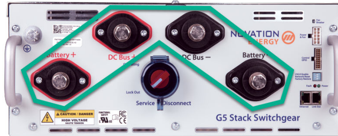
Figure 54. Battery Stack and DC Bus Connector Lugs
