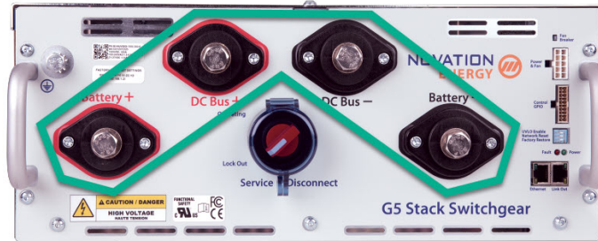
Figure 41. Battery Stack and DC Bus Connector Lugs
